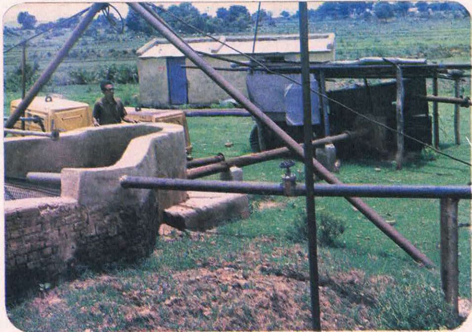
A View of Surface Installation at Ramjibanpur P. S. Project - ECL (MT/36)
