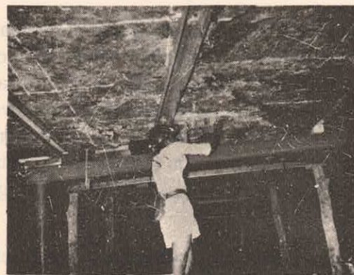
Junction support at GDK-9 with steel girders set on steel props, at cross channels with roof bolting (MT/9.3)
