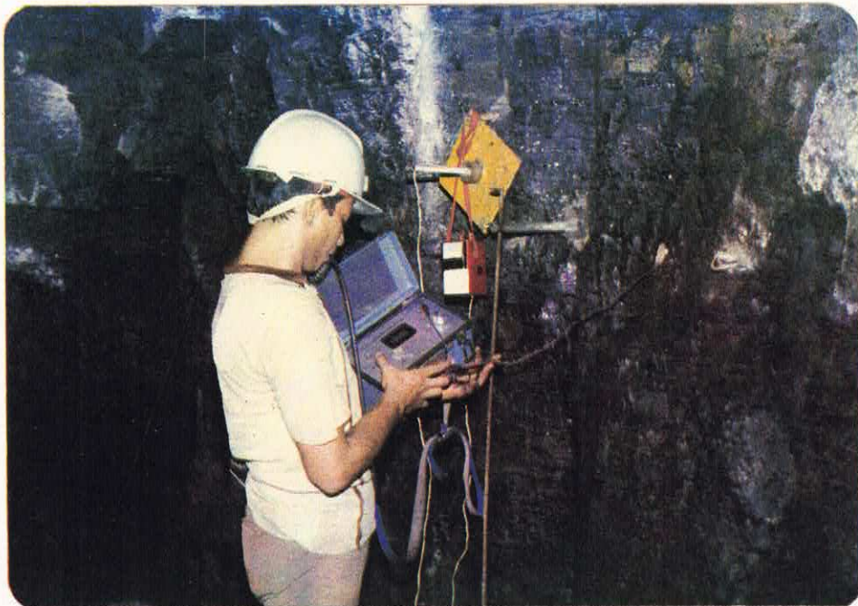
Vibrating wire stress capsule and borehole extensometer in pillar for stress & deformation study (MT/9.3)
